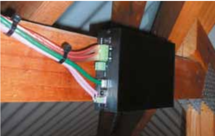
Amplifier installed in roof space
